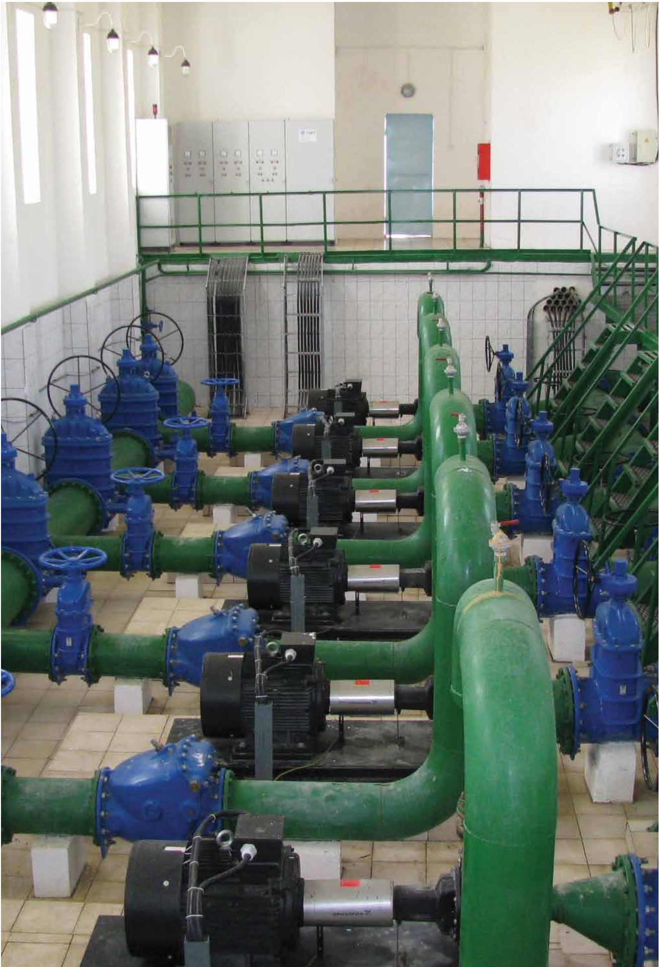
AVK valves installed in the Gokje-Yalkym pump station, in Turkmenistan
