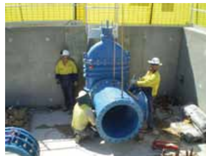
Series 54 DN 750 gate valves during installation in Sydney desalination pump station Ian Simpson, AVK Australia Pty Ltd
