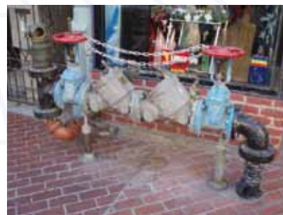
AVK gate valves installed in San Diego, California Calle Ottosson, ERVEX AB, Sweden
