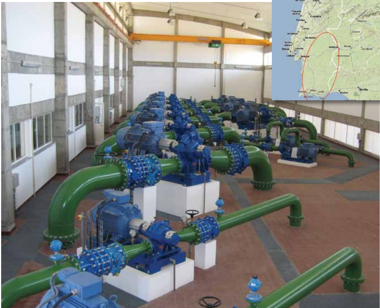
The Pisão pump station is a completed EDIA installation irrigating an area of 2,297 ha. The installation pumps 3626 L/s. (3,6 m 3 /s or 13,054 m 3 /s).
