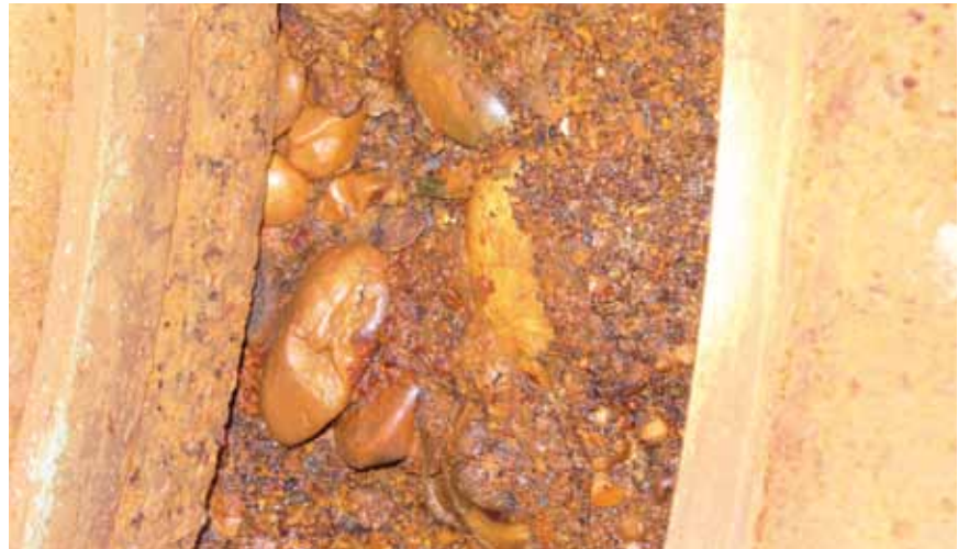
The groove under the closing part collecting debris, stones etc., and this “barrier” prevents a correct closing process in the wedge resulting in a leakage
