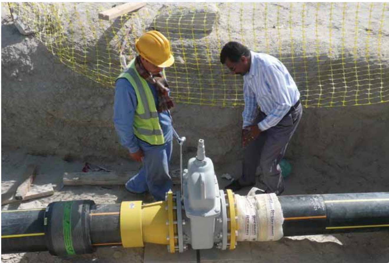
Installation of a Donkin coupling and series 54 gate valve Royce Paul, AVK Middle East F Z E, Dubai, UAE
