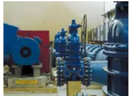
AVK gate valve installed at Kalu Ganga Water Treatment Plant, Sri Lanka.
