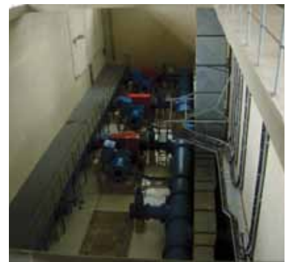
Valves installed three levels below ground level
